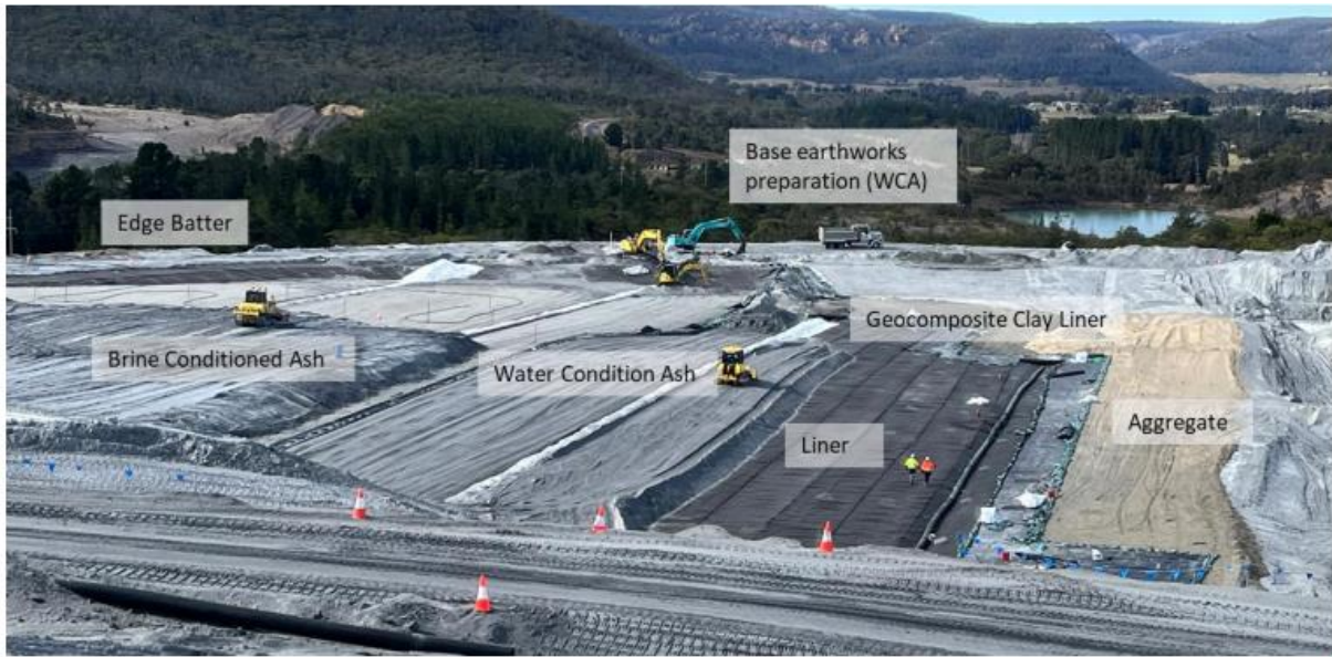
Plate 1 Installation of the leachate barrier in LNAR Stage 1A (Photo taken during Q3 2022)
